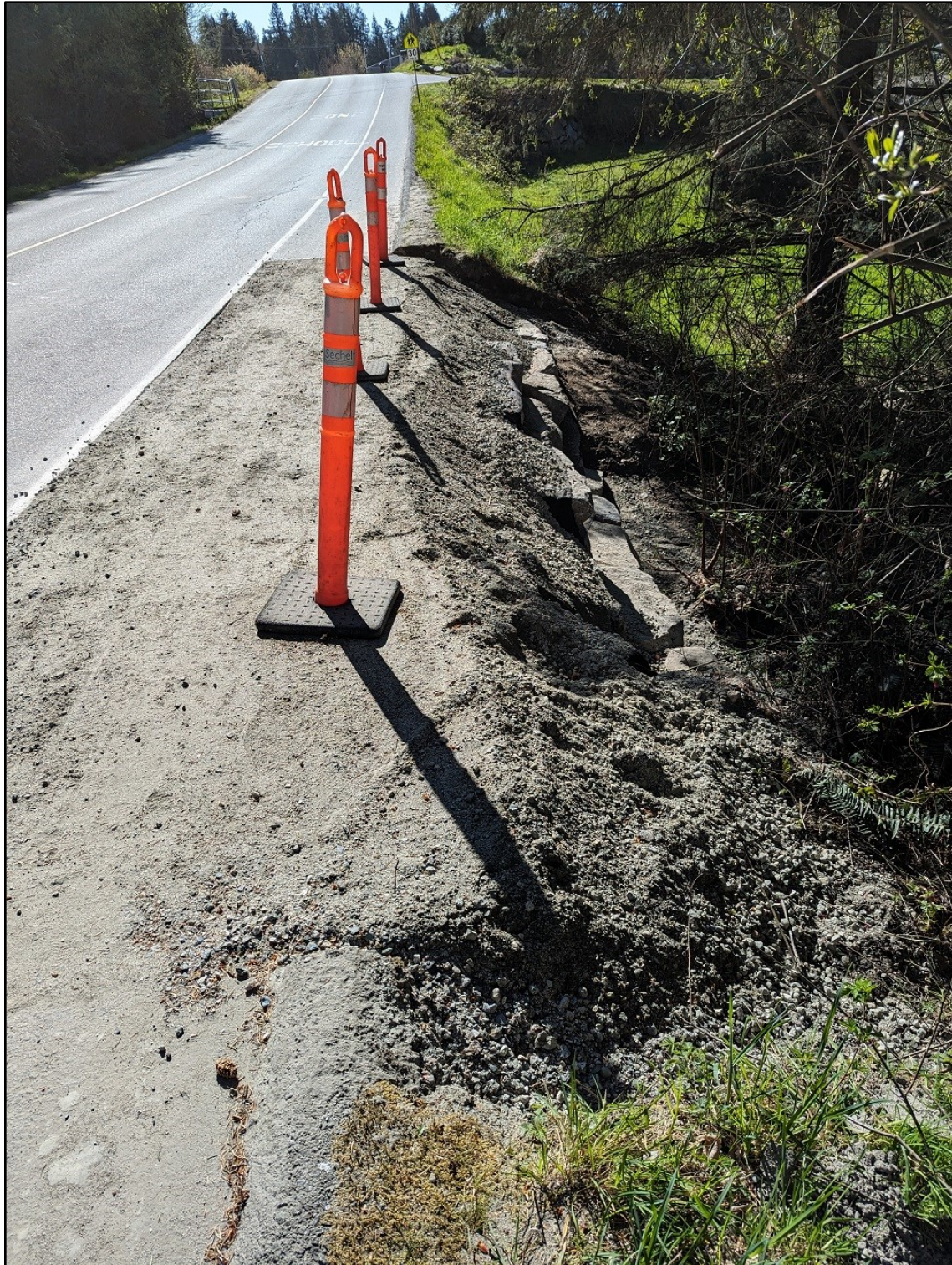
Photo 16: Recently repaired damage to road fill over culvert, Norwest Bay Road.
