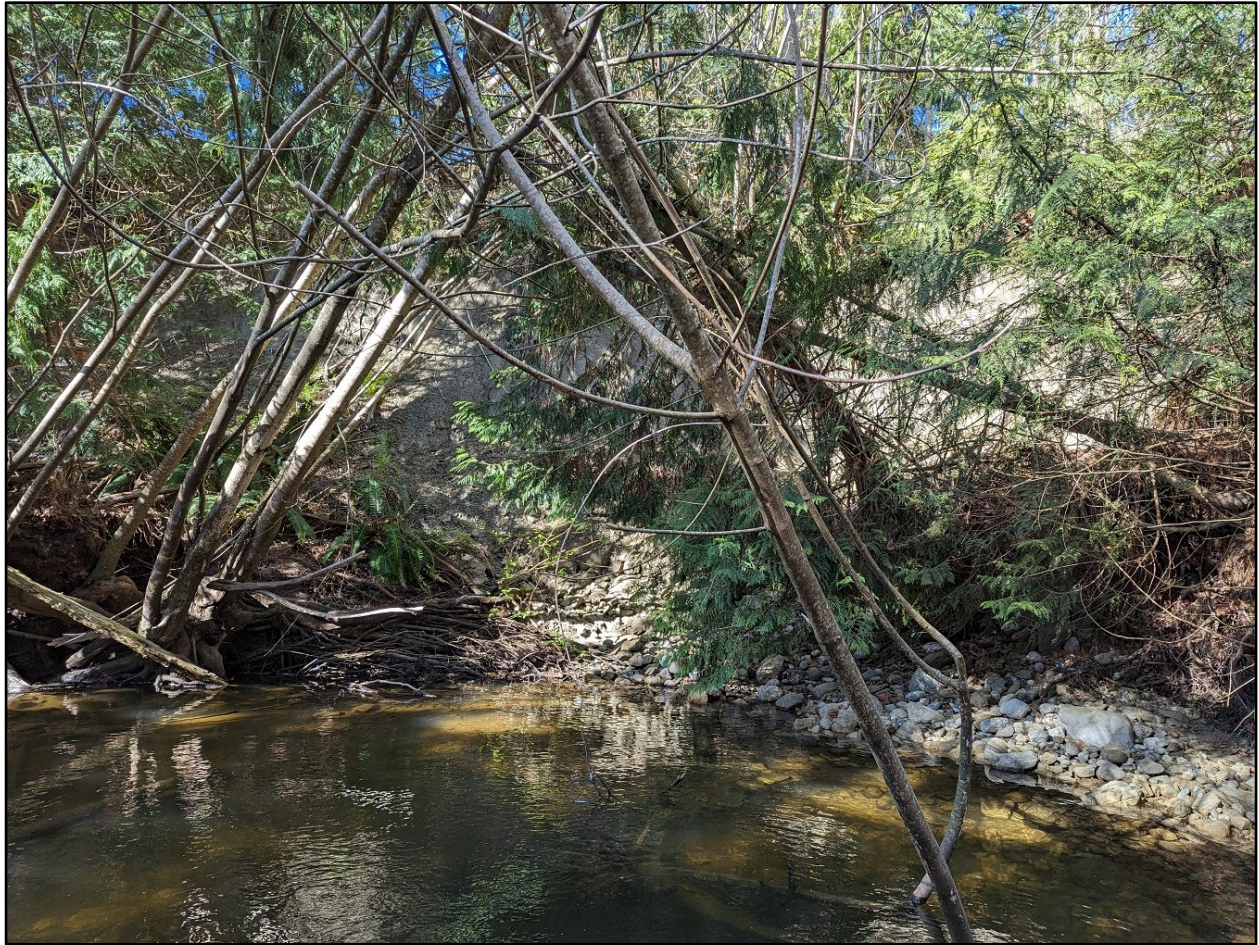
Photo 5: Bank erosion and slump deposit where Norwest Bay Road culvert directs flow against bank.
