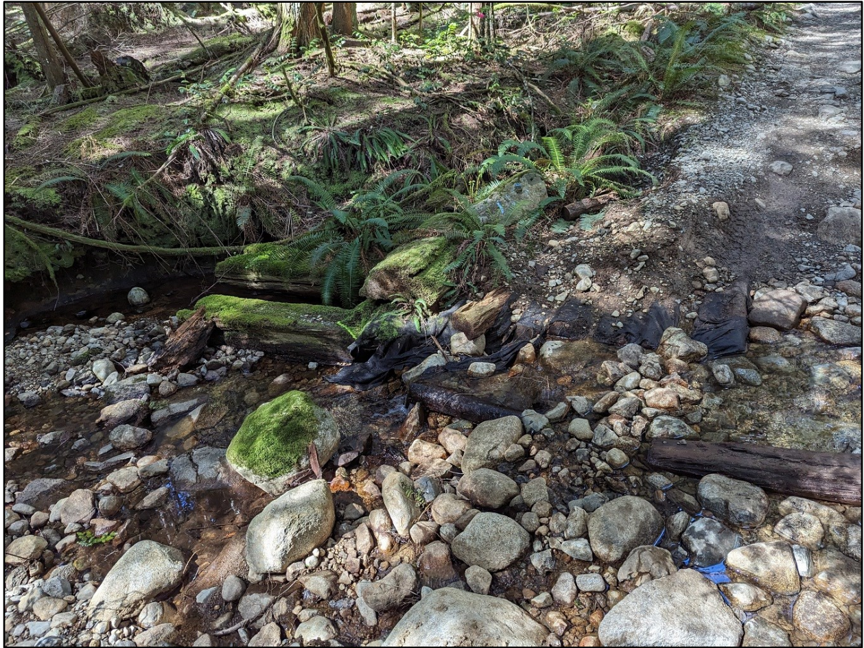
Photo 15: Damaged wood box culvert near outlet of Crowston Lake.
